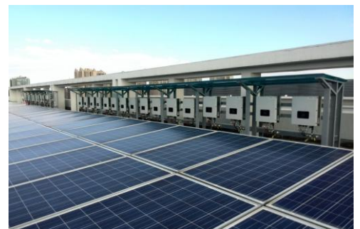
18MW, Huawei Factory
